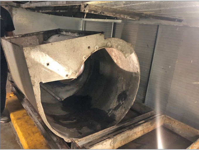
Old Blower Housing Disassembled
