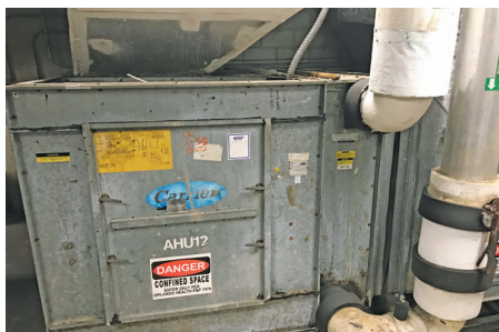
Air Handler Unit (AHU) Before
